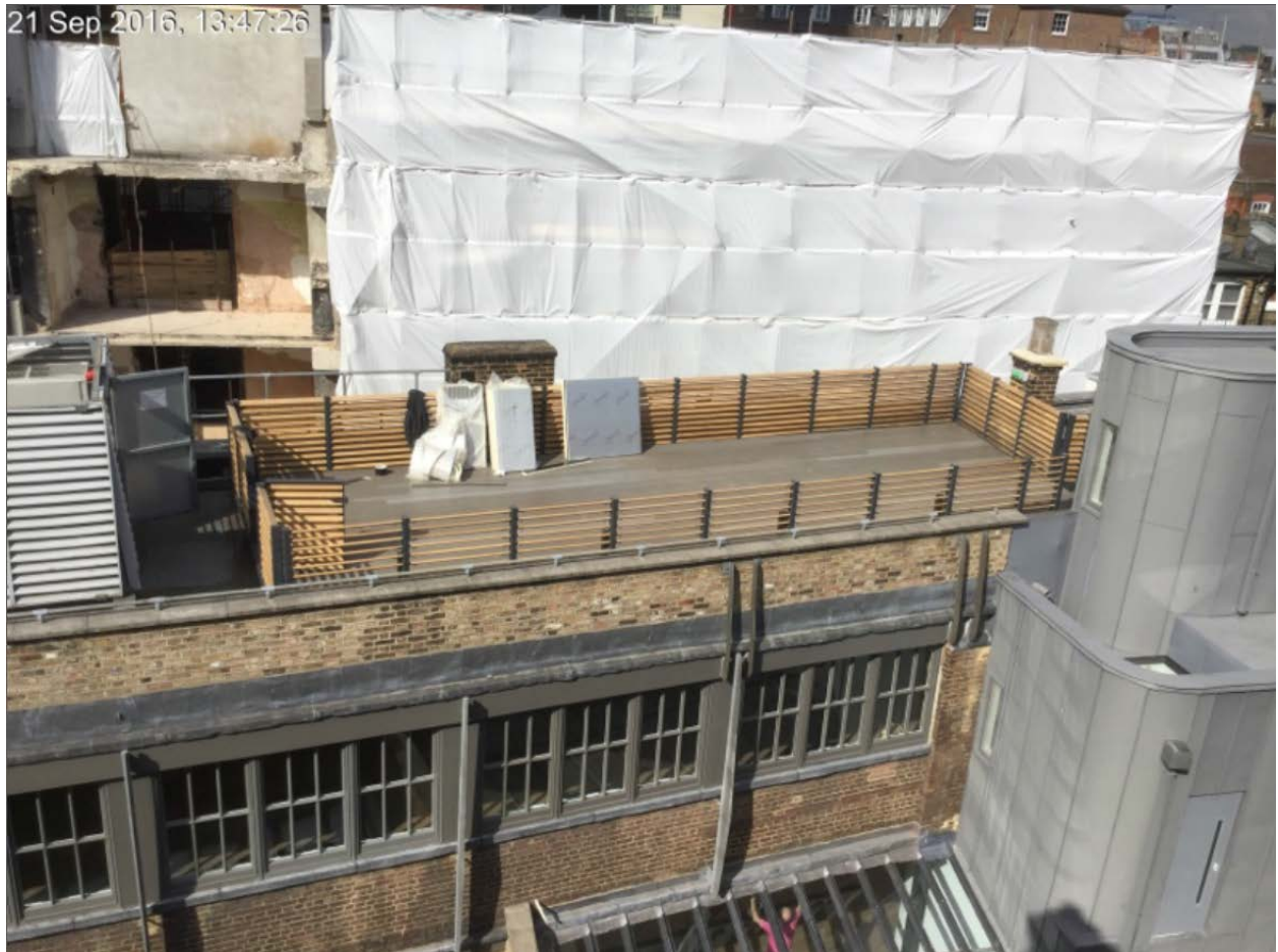
Third floor flat roof of application site as seen from upper floors of properties on Beak Street.
